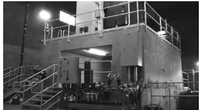
Inside the plant at Juniper Ridge
